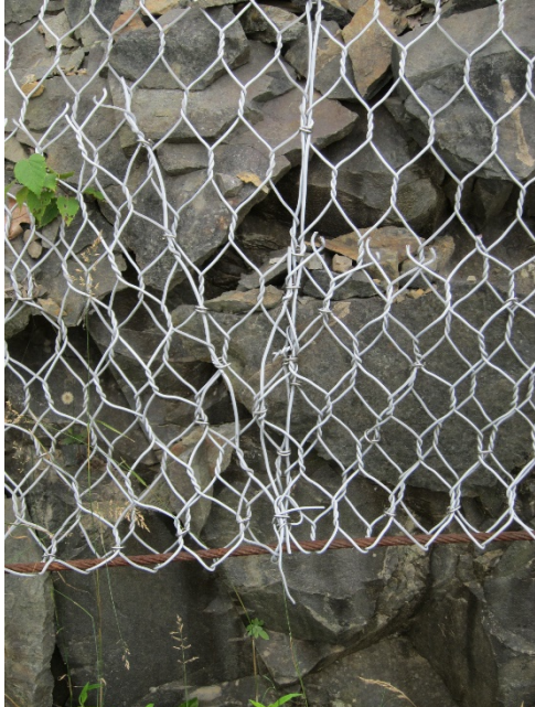
Figure 3. Double Twist wire mesh (gabion mesh) with low tensile strength steel (i.e. 400 – 500 N/mm 2 ) shown protecting a rock slope.
