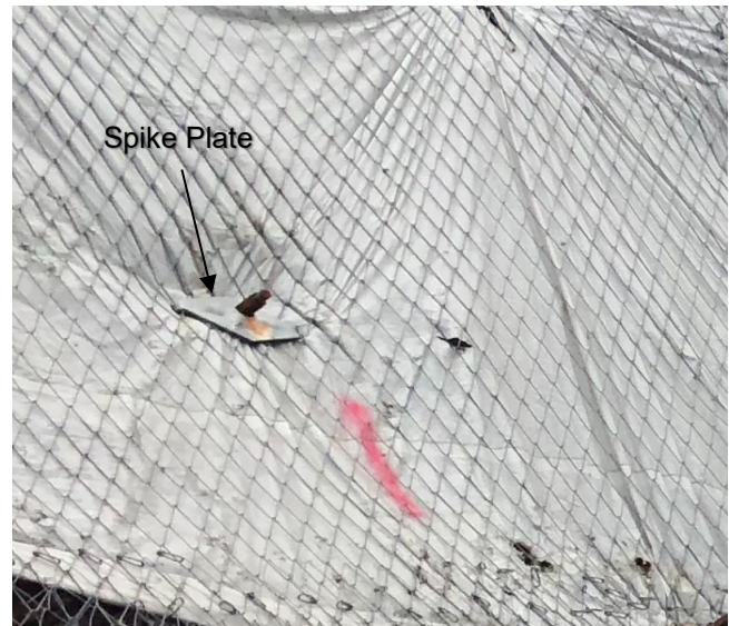
Figure 4. High-tensile G65/3 TECCO wire mesh and TECCO engineered TECCO spike plate used to secure the high-tensile steel wire mesh to the slope. Soil anchors are 25 mm, grade 75 Dywidag.
